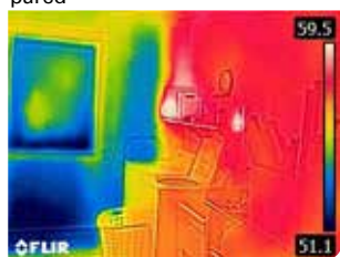
Pared exterior sin aislar
