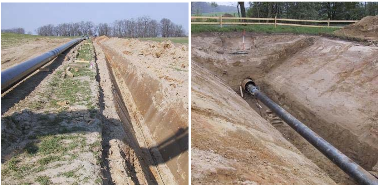
Fig. 5 : Construction phase of a buried brine pipeline in the north-east area of Berlin. The fiber optics cable is placed in the sand at the 6 o'clock position about 10 cm underneath the pipeline .
